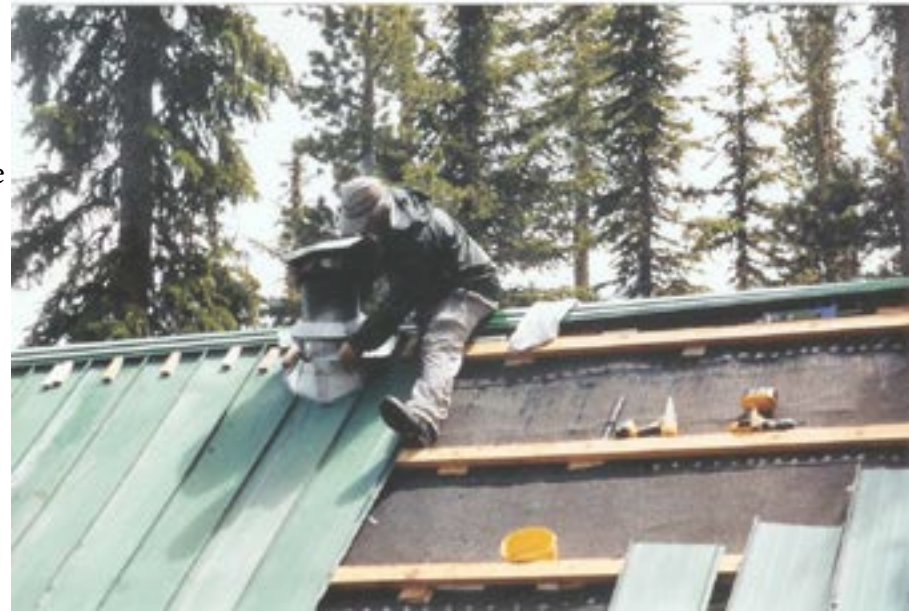
Steve Niday flashes the stove pipe
